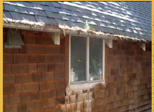
Accumulated fuel in rain gutter.
